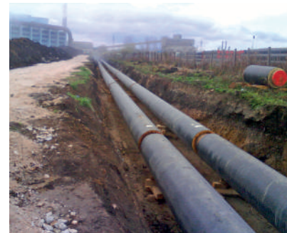
New insulated pipes
