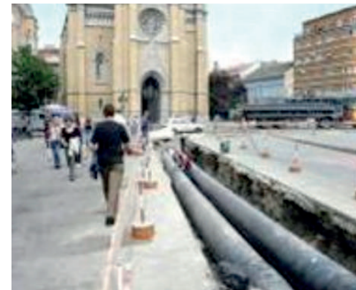
New insulated pipes
