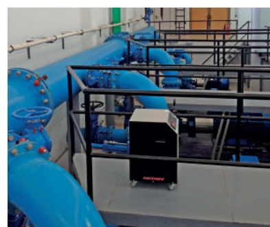
Loznica pumping station
