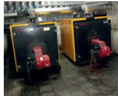
New efficient boilers
