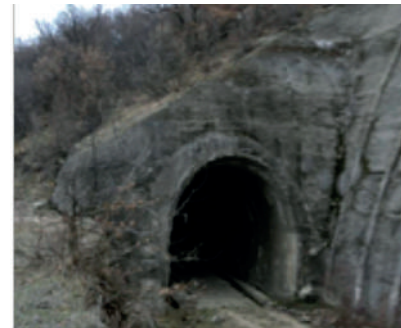
Old derelict tunnel on Beljakovce – Kriva Palanka section for upgrade for speeds up to 100 km/h
