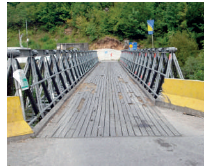
The existing bridge at the border crossing shows the need for upgrade
