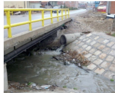
Raw sewage discharge in town centre
