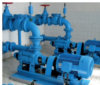
New water pumps for water supply at Doboj
