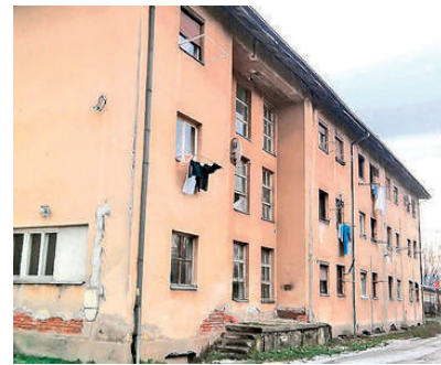
Earthquake damaged block to be replaced
