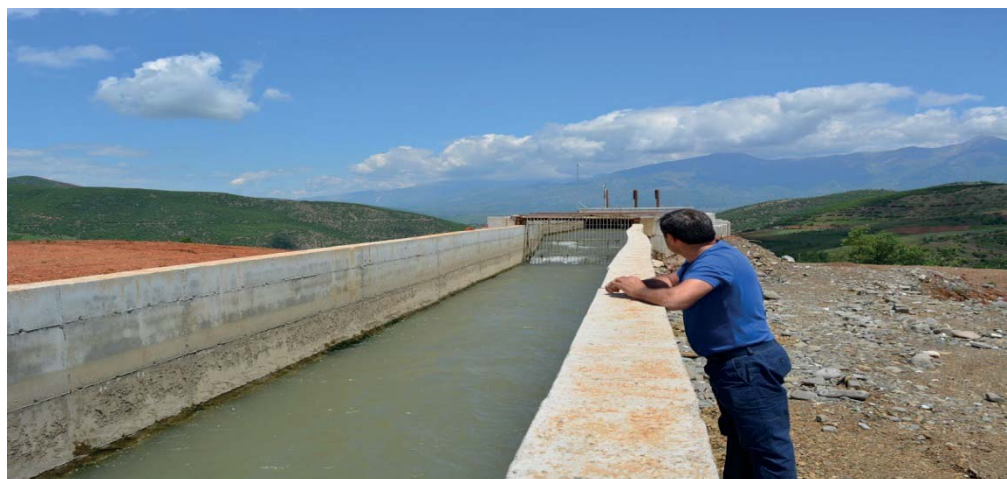
Small Hydropower Plant in Librazhd, Albania.
