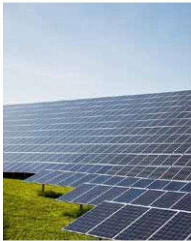
Kosovo: new solar plant accelerating green transition March 2024
